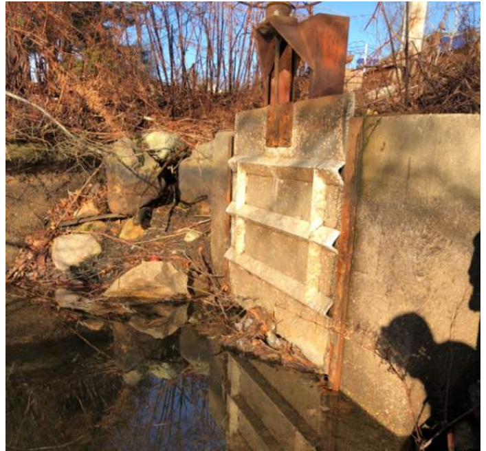
Photo 7 Gates Street culvert, rusted OCS gate
