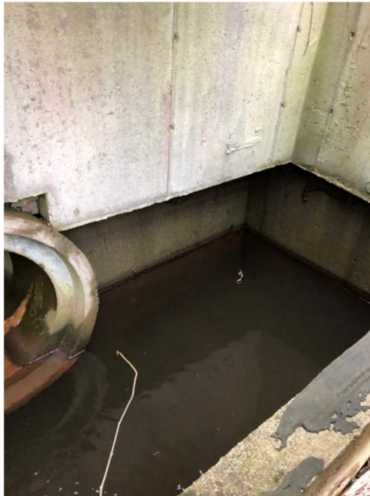
Photo 16 Garvey Road culvert, inlet dislodged OCS superstructure
