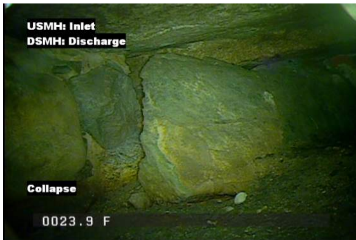
Photo 1 Hartford Street culvert, interior collapse
