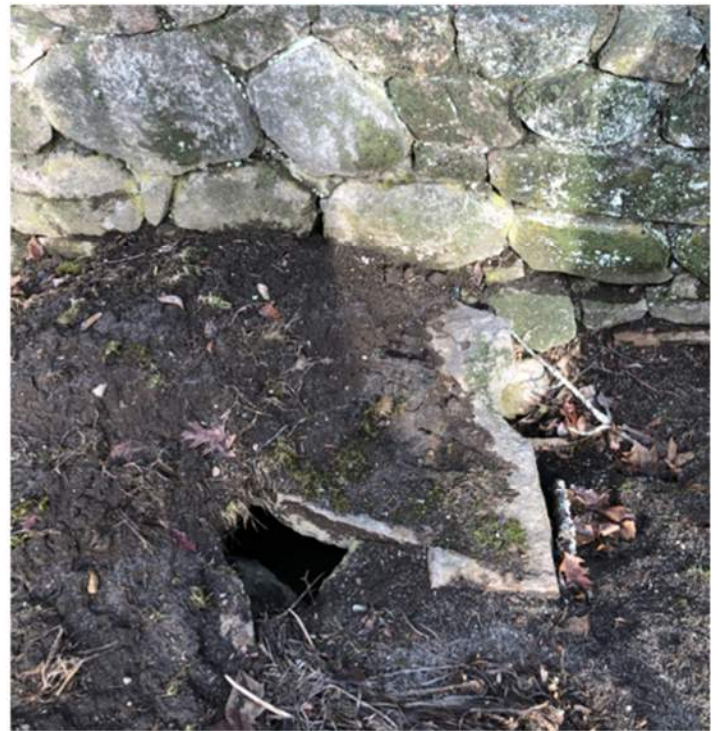
Photo 11 Salem End Road culvert, exterior hole in culvert roof
