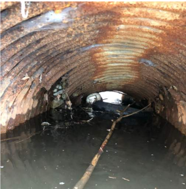
Photo 4 Waushakum Brook, deformation, second from left culvert
