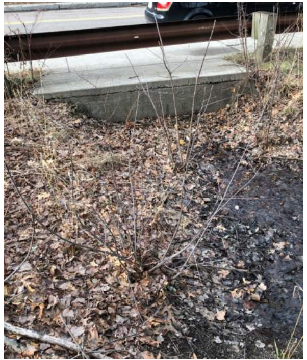
Photo 3 Herbert Street culvert, upstream blockage
