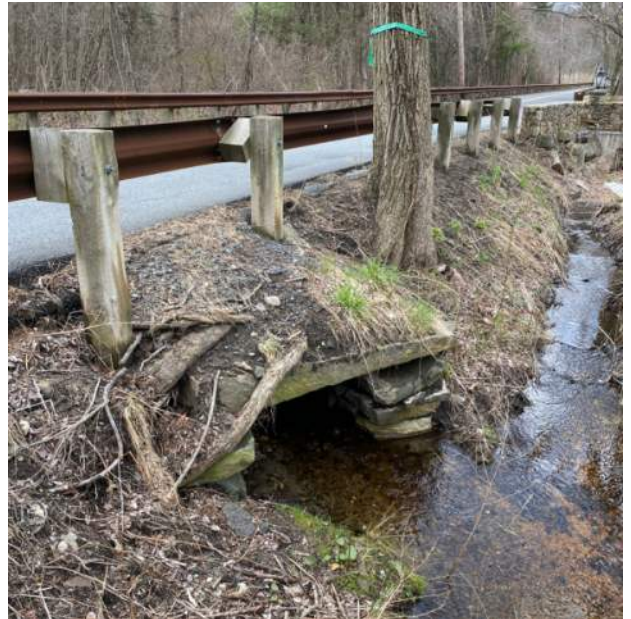
Photo 9 Wayside Inn Road culvert, downstream embankment erosion
