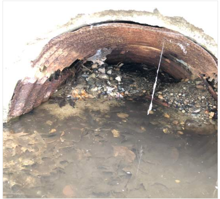
Photo 5 Waushakum Brook, interior collapse in left culvert
