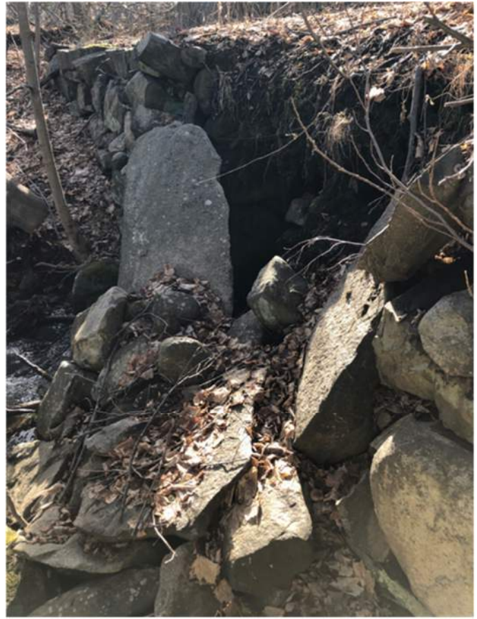
Photo 14 Badger Road culvert, downstream headwall collapse
