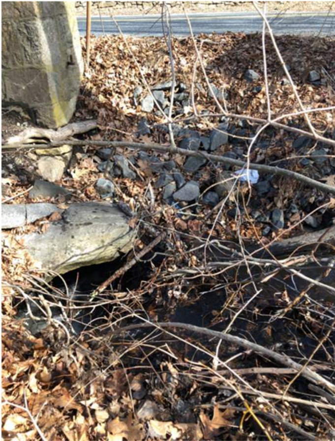
Photo 13 Badger Road culvert, upstream headwall collapse and erosion
