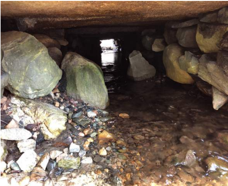
Photo 8 Wayside Inn Road culvert, fallen interior stones
