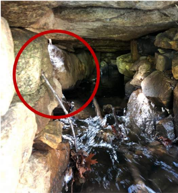
Photo 10 Salem End Road culvert, interior stone roof collapse
