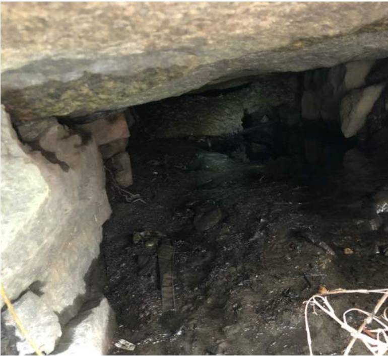
Photo 2 Herbert Street culvert, interior collapse
