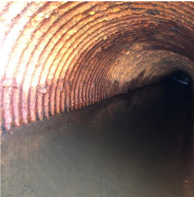
Photo 6 Gates Street culvert, interior deterioration
